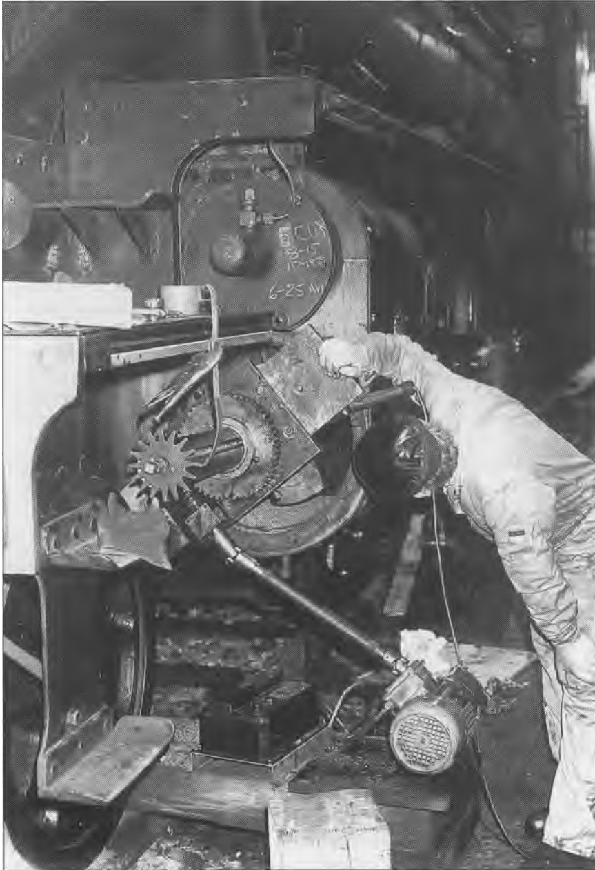
Ian Storey care fully watching the reboring of the left hand cylinder of the K1 on 23.1.02 (John Hunt)
