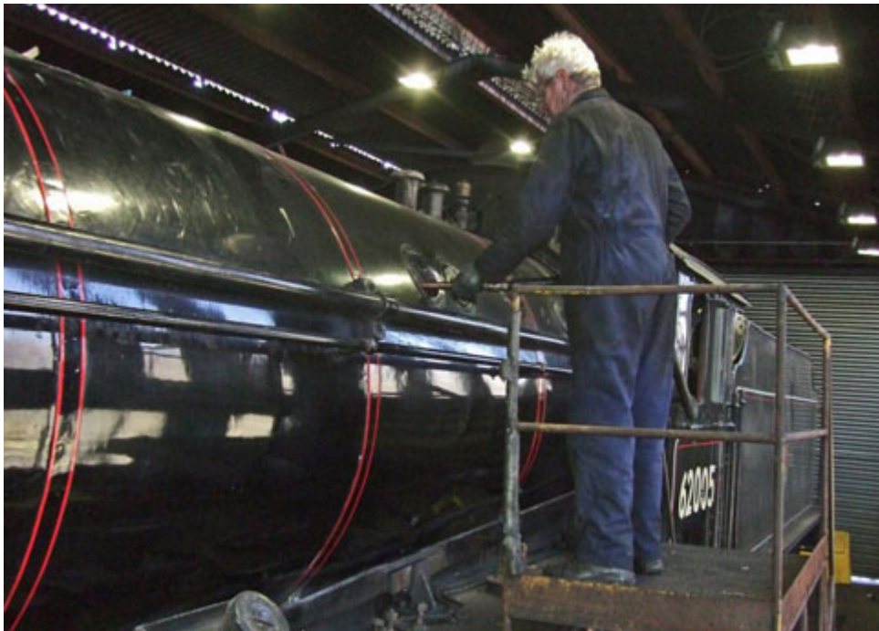
Dave Donegan washing out the K1's boiler at Grosmont on 19 th April (Colin Smith)
