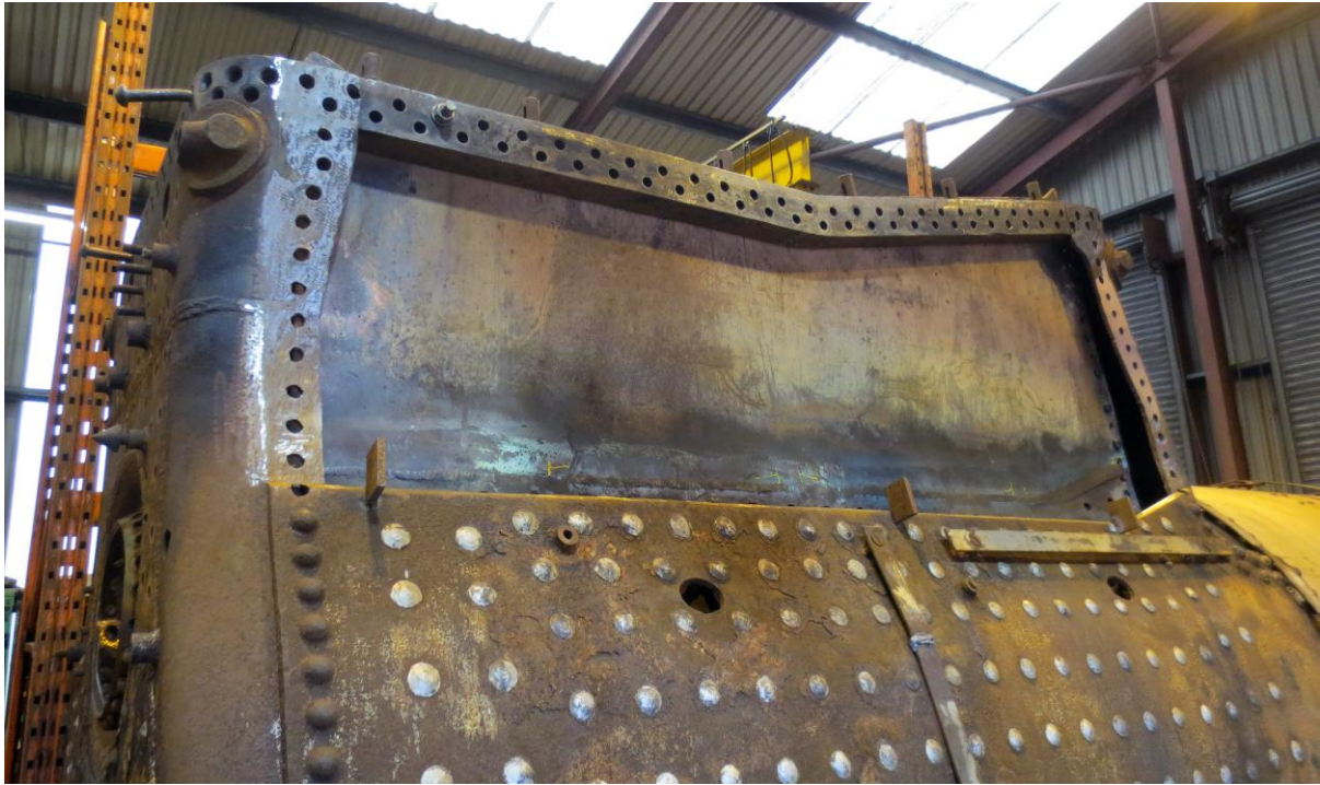
The same sheet viewed externally and showing the foundation ring in place (John Hunt)
