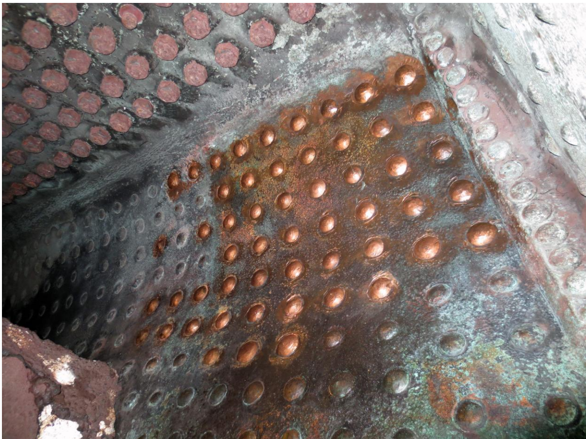
The 53 new side stays in the top RH side of the firebox on 12 th September; note the crown stays and the top of the brick arch on the left (John Hunt)
