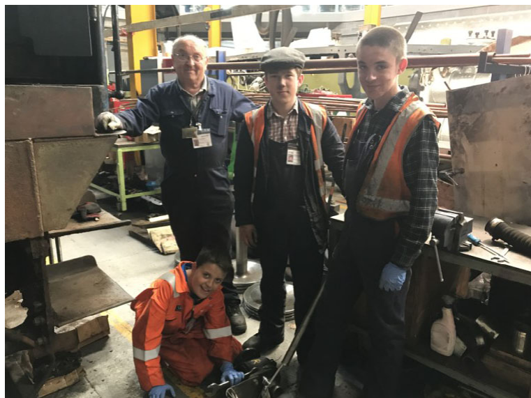
The above photo shows (left to right standing) me, Ed Murray, Ethan Humble and new JV Luke Perry (sitting) wrestling with the Sir Nigel Gresley tender water valve fixing bolts on Saturday 5 th August 2017. Luke is wearing one set of the overalls which Steve Hyman donated to me for future use by our Juniors. Many thanks to Steve! (Will Harrison)
