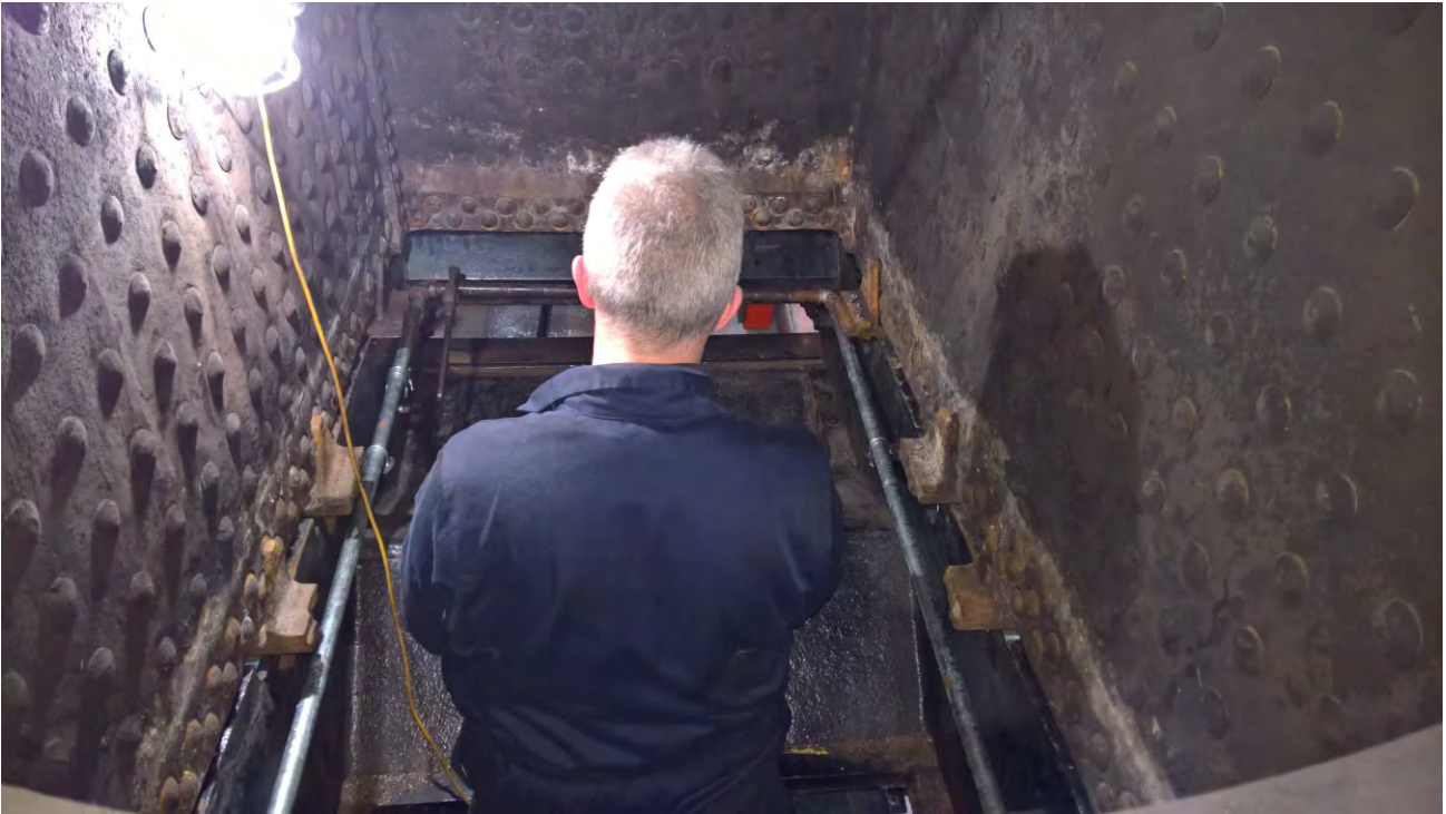
Paul Swainston fitting the new pipe work for the ashpan sprinkler system, which is clearly visible in this view looking down into the ashpan (Richard Pearson)
