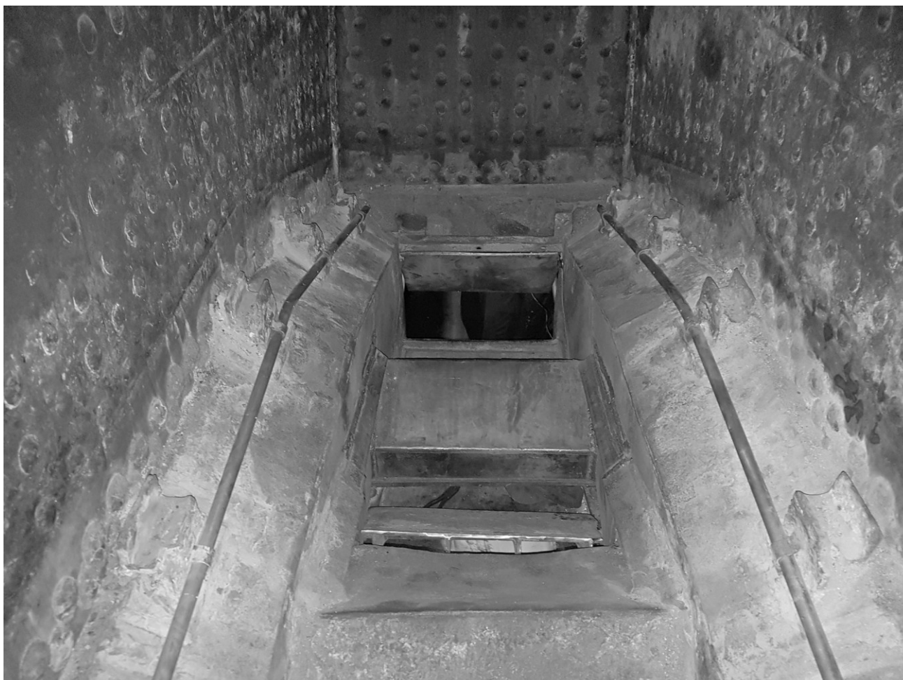
The new platework in the K1's ashpan and the pipe work for the ashpan spray (Rowland Bingham)
