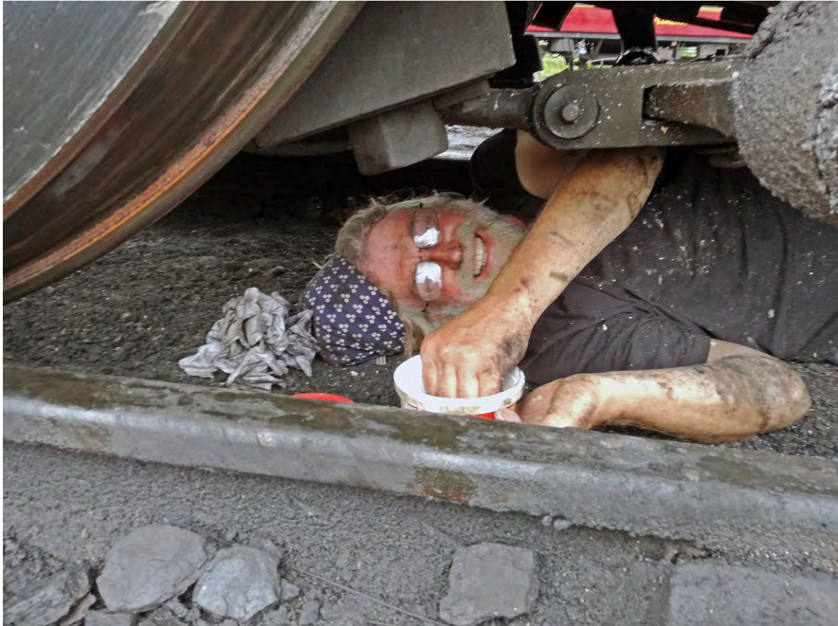
Getting down and dirty: Paul Hutchinson applying fireclay to seal the hopper ashpan in order to reduce fire risk on 26 th June (Saskia van Schip)
