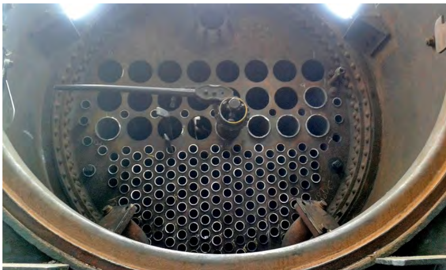
With the small tubes in place, the large flue tubes in the process of being fitted on 13 th June (Bill Dobson)
