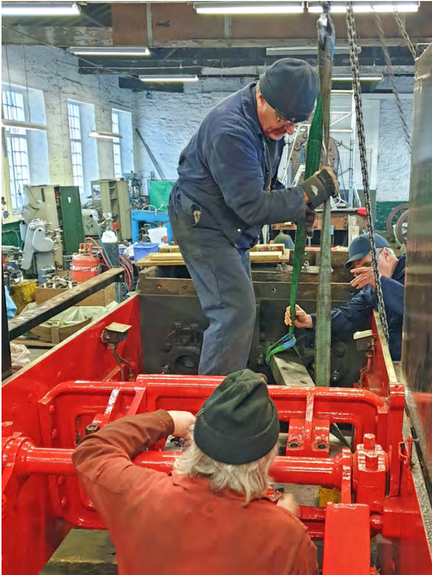
Arthur Jenkins controls the lowering of the slide bar whilst Tim Williamson and Norman Wells guide it past the obstructions. Out of sight is John Jones pulling the chains (Nigel Hall)
