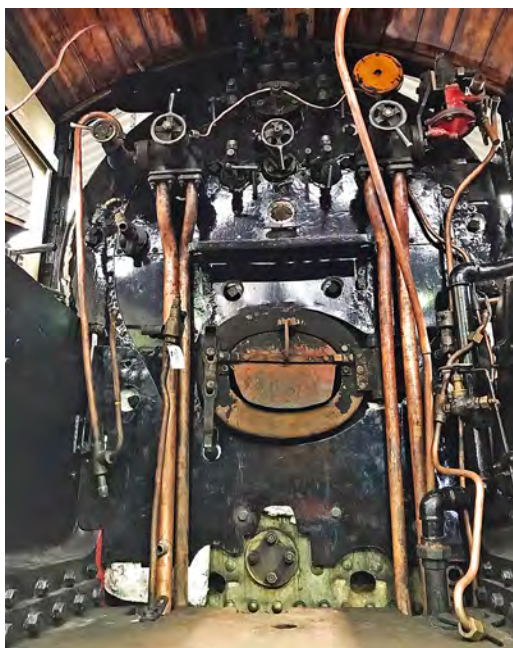
On 26th May, most of the cab fittings and pipework are complete in the Q6 cab (Ian Pearson)
