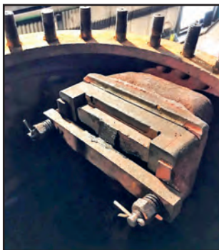
Left: The new stud fitted to the dome Right: The J27 regulator in the dome with the J-pipe hidden beneath it in the shadows (both Ian Pearson)
