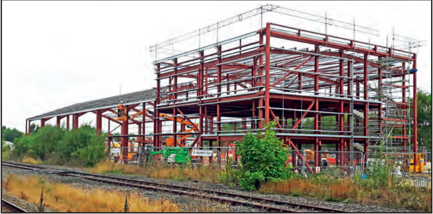
The new A1 Trust building on 18th August. In the left foreground is the Darlington to Bishop Auckland line (Richard Barber)
