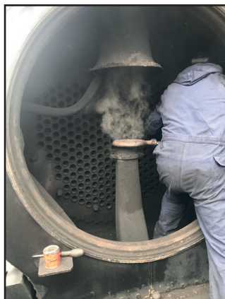
Top: the broken blower ring. Bottom: Paul Wickham fitting the new pipe and ring (both Ian Pearson)
