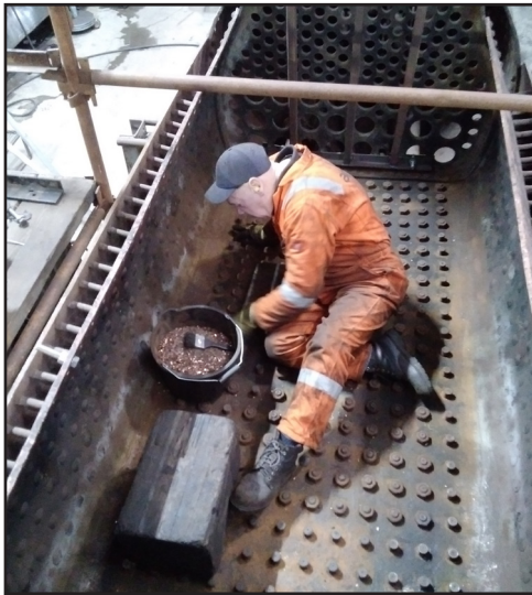
Steve Gibson removing swarf and general debris from the crown sheet after removal of the firebox sides and the barrel with the defective section removed on 12th January (Paul Hutchinson)
