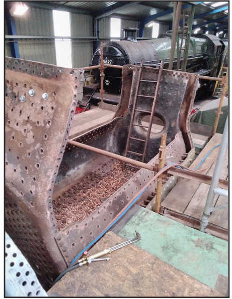
A general view of the K1 firebox on 5th January with the sides and foundation ring removed on 5th January (Paul Hutchinson)
