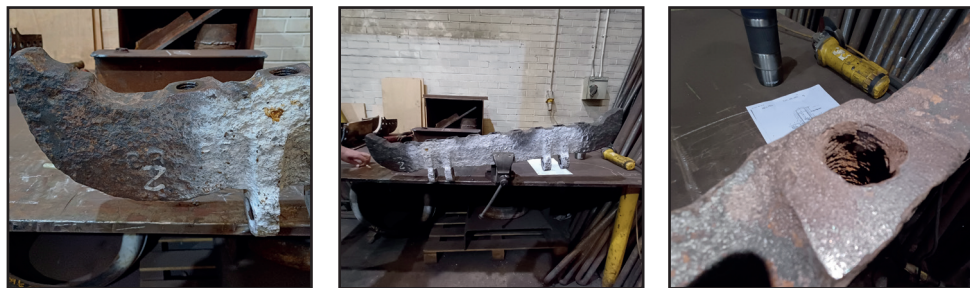
One of the girder stays, pictured upside down, showing the extent of corrosion and, on the right, the badly wasted threads (all Dave Pennock)
