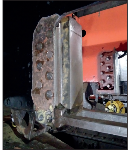
The refitted trailing wheelset horn blocks machined and refitted on 7th November (Paul Hutchinson)
