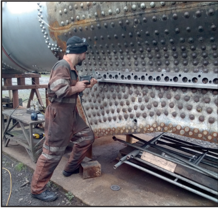
Chris Henwood drilling an expansion bracket stud pilot hole on 17th October (Paul Hutchinson)
