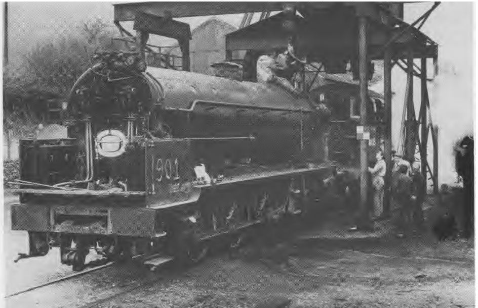
Trevor Mussett guides the refitting of the ars chimney on 22nd April helped by Richard Pearson, Gordon Wells, Nigel Hall and Maurice Johnson. (John Hunt)
