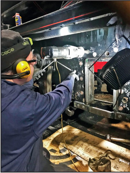
George Bee reaming out the RH side horn block bolt holes using the magnetic drill on 22nd January (Ian Pearson)
